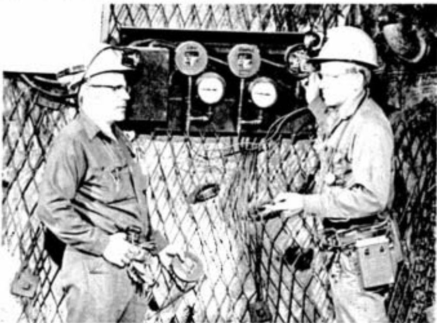
In the 3,800 level shaft station, electrical foreman, Gene Liciotti, left, and electrical leader, Richard Laframboise, check the water reservoir's high and low pressure sensors.
