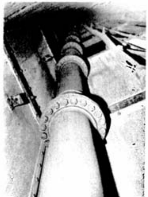
In the shaft compartment, with its bottom end located at the 3,800 level of the mine, this is the 100-foot long, 14-inch diameter water system reservoir.
